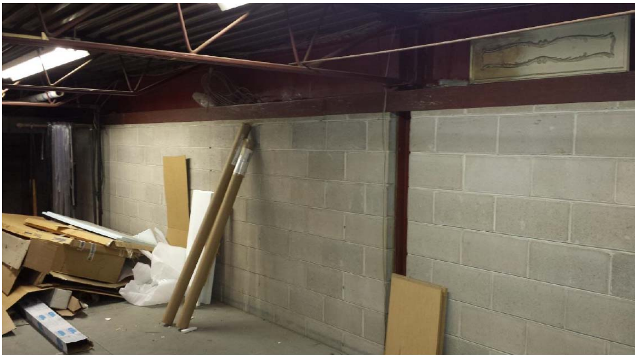
Photo No. 3: Non-load bearing masonry wall between Bays #1 and #2. Similar construction throughout other bays.
