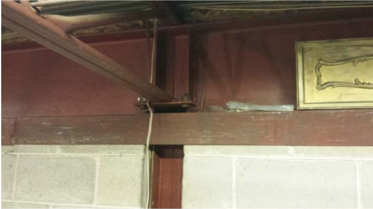
Photo No. 2: OWSJ spanning to steel beam and column between Bays #1 and #2.
